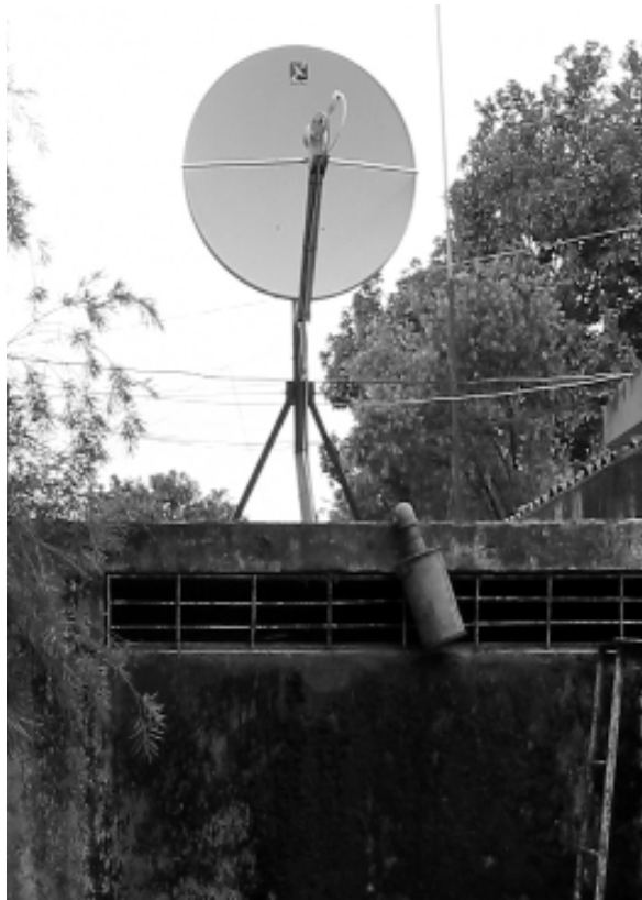
Dishing up the Internet – the ANGONET VSAT satellite system, sending and receiving broadband for NGOs in Huambo.
